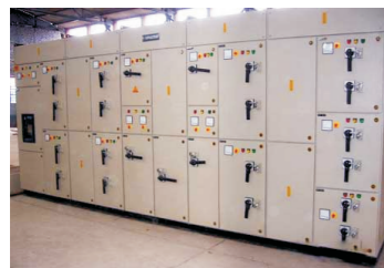
Distribution Panel (MDP)
