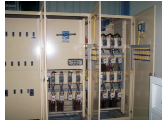
Main Distribution Panel (MDP)
